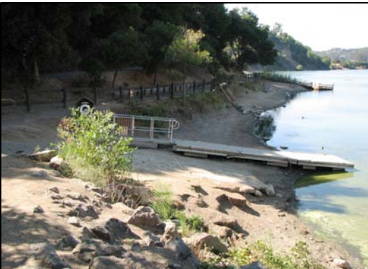
Floating dock at low water elevation & eroding bank undermining trail
